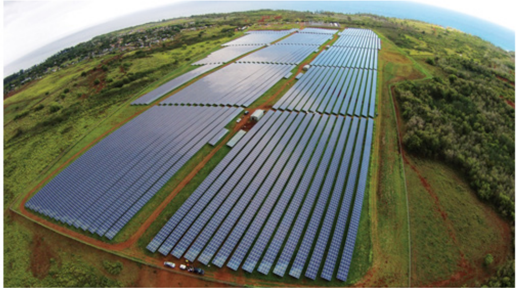
When KIUC's $50 million, 12 megawatt solar farm in Anahola comes on line later this year, it will be the largest in Hawaii. "I think we added an extra panel so it would be larger than our Koloa Mill project," jokes CEO David Bissell. Photo: Courtesy of KIUC
