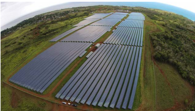
The energy cooperative on Kauai oversaw the massive Anahola solar project.
